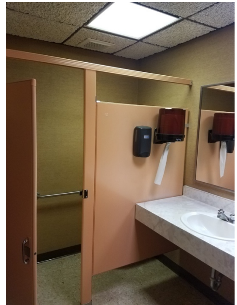
Outdated women's restroom.
